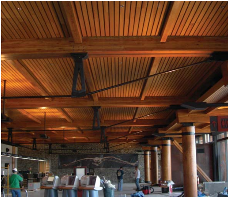
ACCOUSTICAL CEILING of the newly renovated ticketing hall at Jackson Hole Airport, Grand Teton National Park, Wy., was manufactured from cypress rather than Douglas fir. (Photo by Rulon Co., St. Augustine, Fl.)
